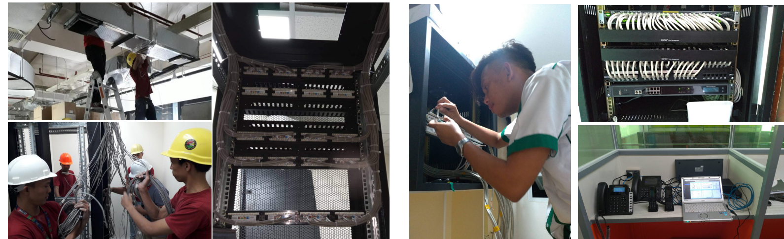
Structured Cabling to a Australian offshore staffing company Makati, Metro Manila | 2018
