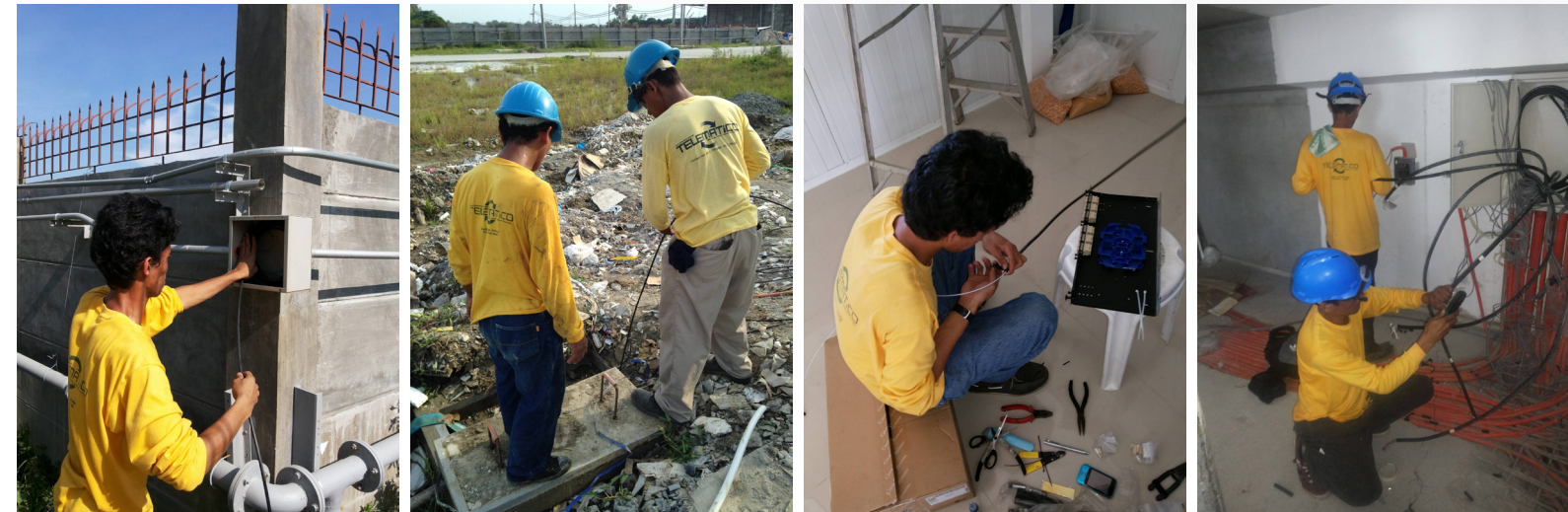
Fiber Optic Installation to one of the biggest food manufacturing company in the world Ilocos Norte Province | 2013
